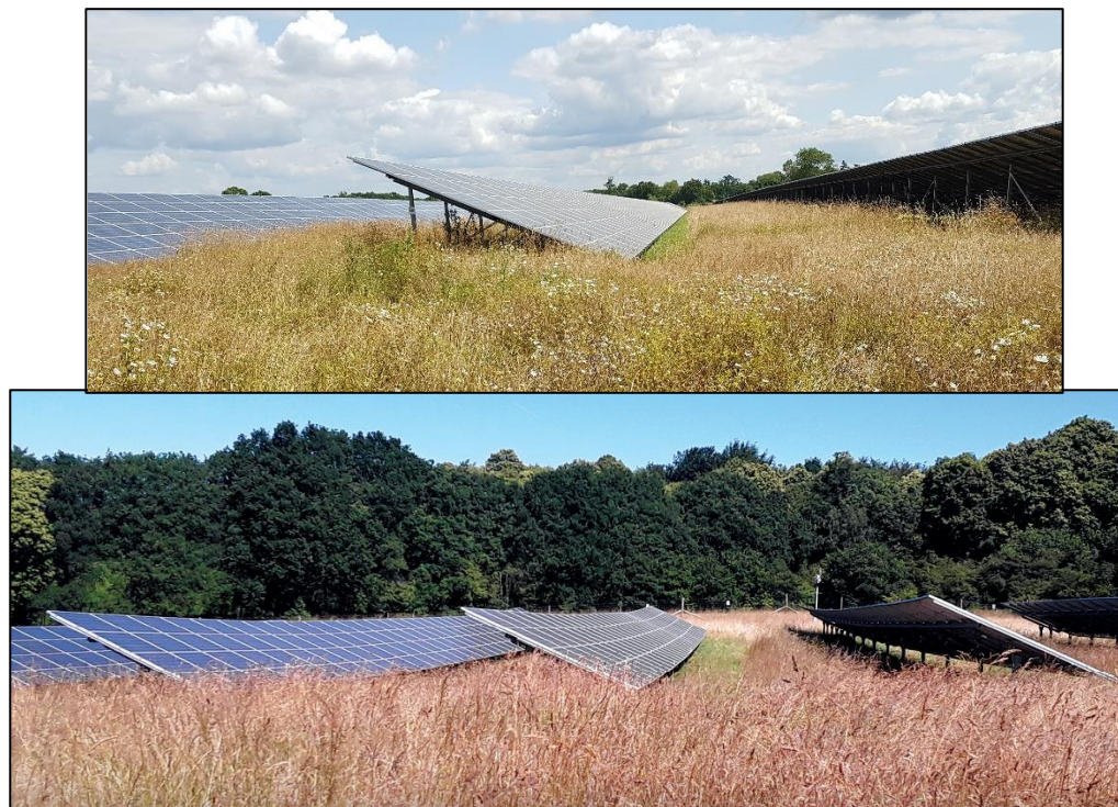
Figure 4. Photographs to show a 'Shade Cut' along the first 1m of grassland from the toe edge of the array, leaving flowering and seeding meadow grassland elsewhere.
